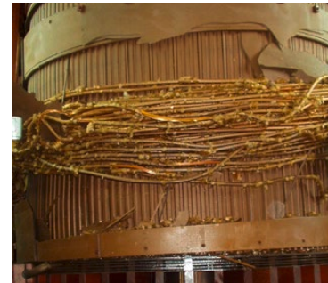
Collapsed tap winding
