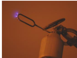
Corona Discharge – 400 kV Arcing Horn
