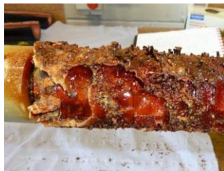
Insufficient Mastic Around 33 kV XLPE Connector
