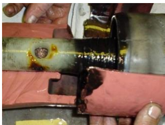
Failure of 110 kV Transformer Termination
