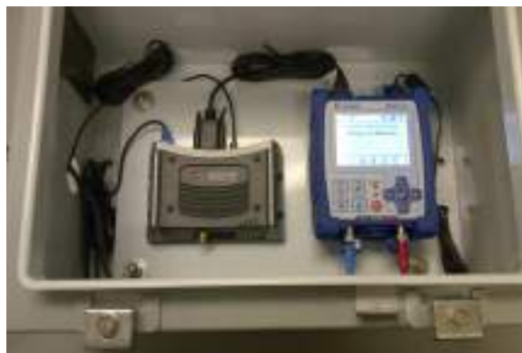
Mounting Panel Installed in the Enclosure
